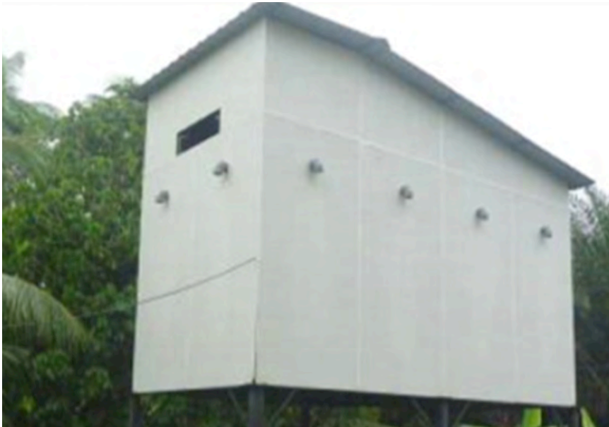
Figure 2. Another house design in Johor that uses Shed Roof and double layer wall with plywood on the inside and plaster board on the outside.
