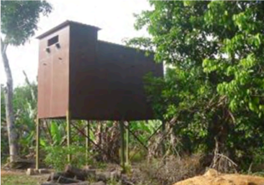
Figure 1. One of the swiftlet houses in Johor that uses the Jack Roof design and plywood board as the main material
