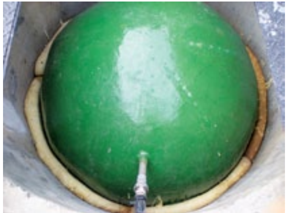
Figure 3. Biogas holder or dome
